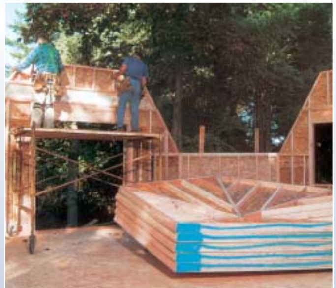
Panels, drilled and ready to install. Workers set the wall top, part of the exterior wall kit for a 35 foot diameter dome on a five-foot riser wall. Clients select their windows and exterior doors locally, providing the rough openings for us to draw and frame. All panels are loaded by hand at ODI, you and three others unload.
