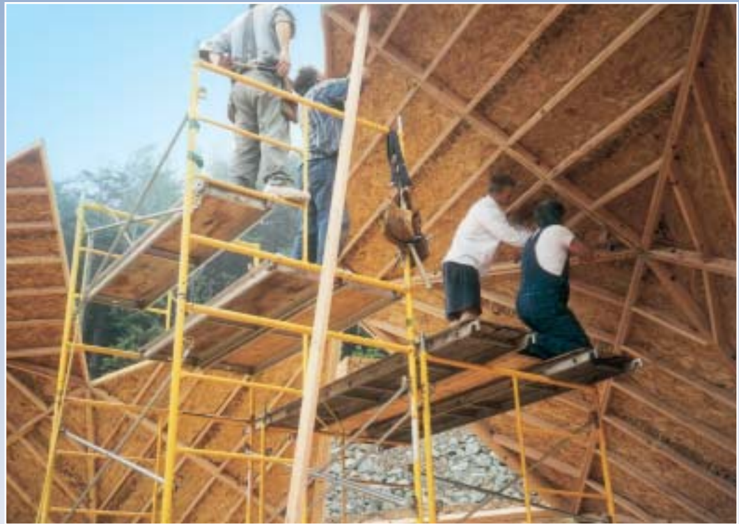
Nearly adequate scaffold for raising a 50 foot diameter, 2 x 4 dome with six volunteers in one day. As many as twenty people are welcome to carry panels, move the scaffold and learn about geodesics.
